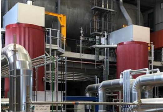
Extra 100 MW electric boiler capacity
