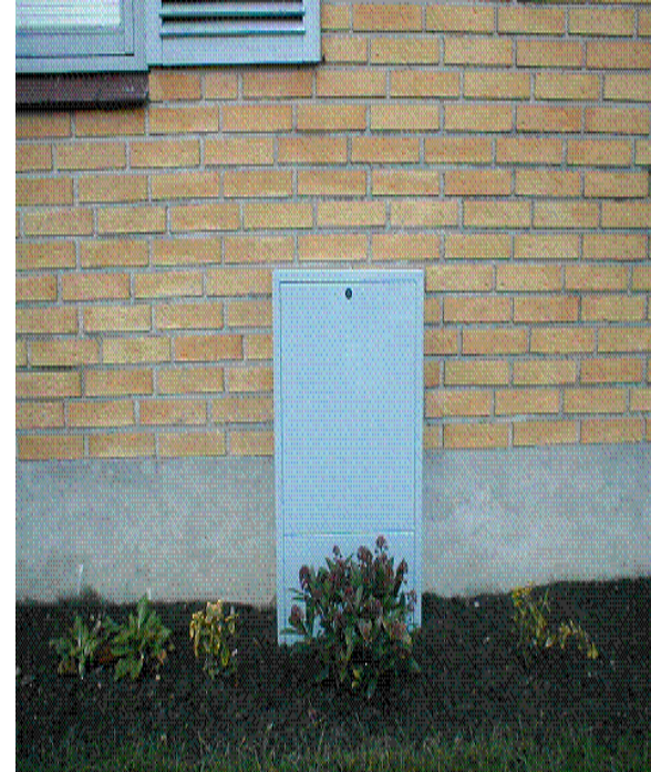
Intersection point cover
