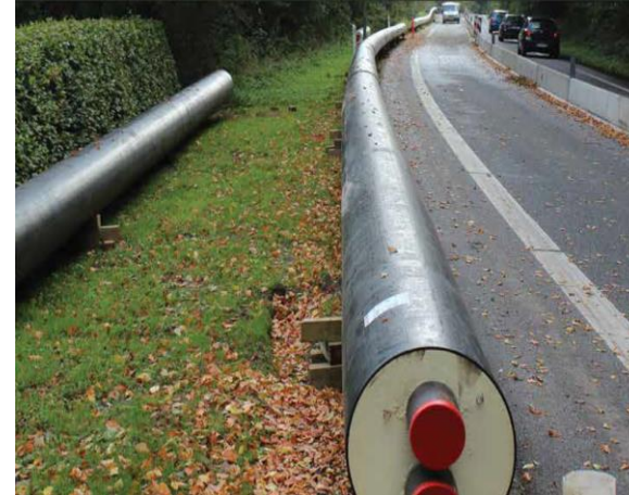
Pipes ready to be dug down on the side of the road
